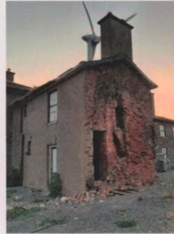
Plate 4-4 Collapsed wall on the south facing aspect of the derelict farmhouse.
