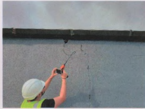
Plate 4-10 Cracks in the cement work being inspected with an endoscope.
