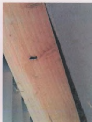
Plate 4-14 Crevice between the wall and sheet metal
