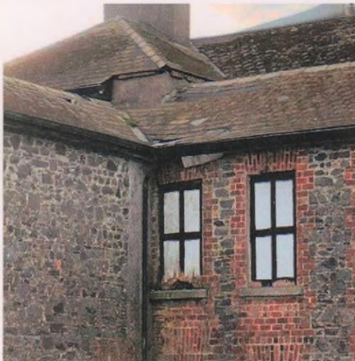
Plate 4-5 Gaps in the slate roof, the soffit, and the boarded window.
