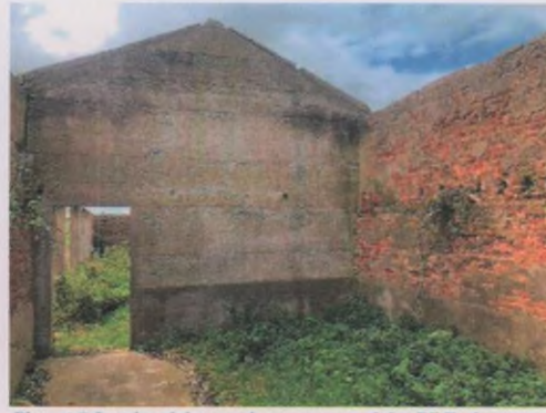
Plate 4-8 Inside of the north-east room of the PRF, showing gaps in the brickwork.
