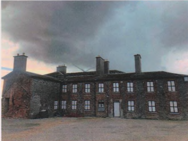
Plate 4-3 South facing aspect of the derelict farmhouse.
